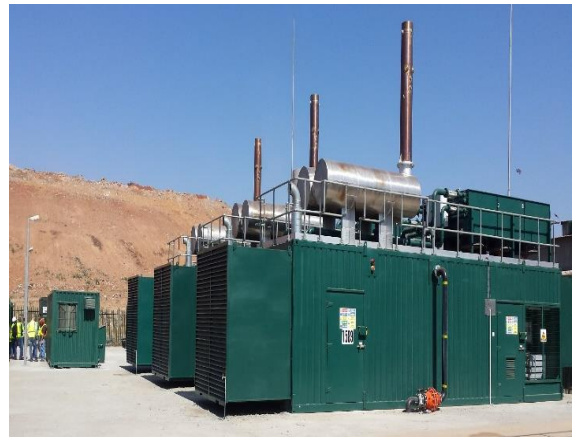
Fig 2: Landfill Gas to Energy at Robinson Deep landfill Johannesburg
